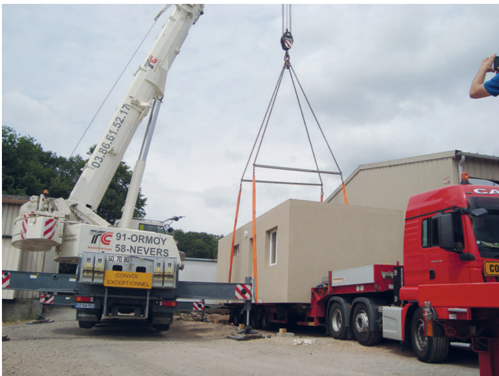
Positioning a modular Cubik Home with Dramix fibre reinforced concrete at its final location
