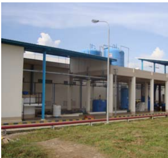
With the new water treatment plant in Karawang, Indonesia, Bekaert will be able to significantly reduce the waste waters of its manufacturing lines.
