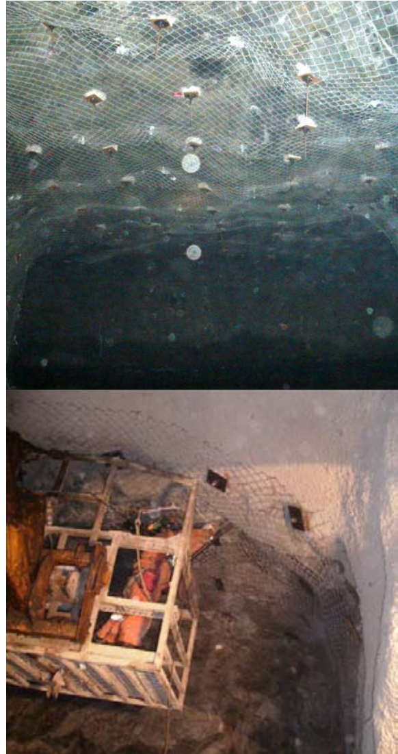
In order to protect miners from rock fall the ceiling and walls of the tunnels in underground mines, through which the ores are removed, are being reinforced with steel meshes.
