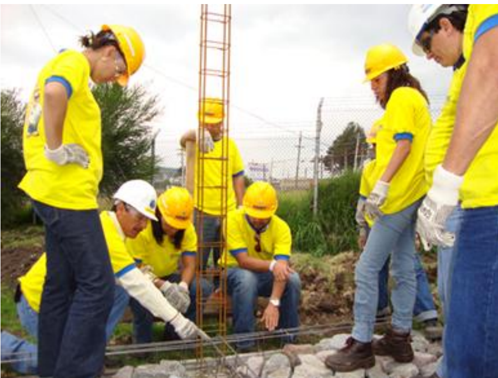
Our plant in Ecuador released the 'Manual para la Construcción'. During workshops construction builders are being trained to build earthquake resistant houses for lower income families.
