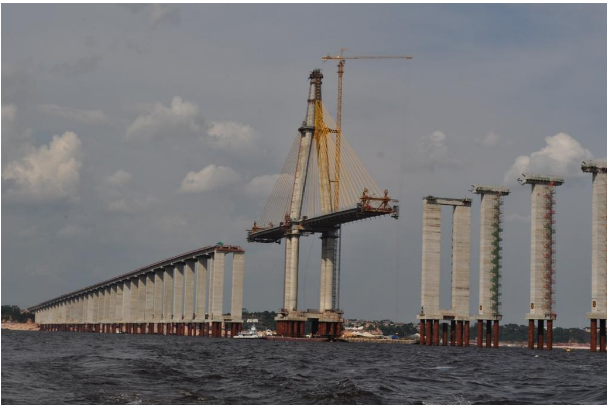
The Rio Negro bridge in Brazil is tensioned by stay cable and prestressed strands from Bekaert's joint venture plants.
