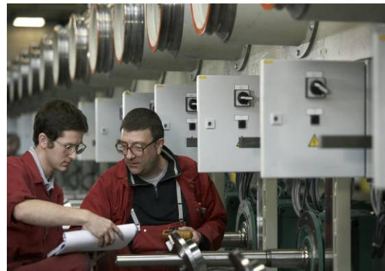
One of the elements that differentiate Bekaert from the competition is the fact that we have our own engineering department on a global level that designs and develops total plant layouts and production lines.
