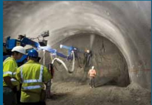
Every year, 120 000 m 3 of concrete reinforced with Dramix®, are sprayed in Peruvian mines.
