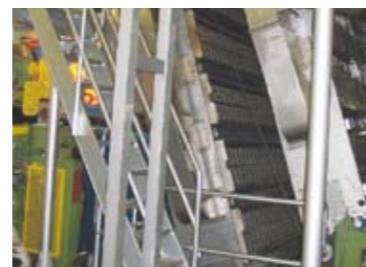
Arjo Wiggins Dettingen - Germany Pre-Impregnated Paper Bekaert UniDryer® V2 Gem 10 520 m/min 7.2 MW 4.16 m
