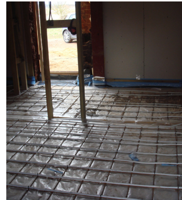
Under floor heating ready for concrete topping
